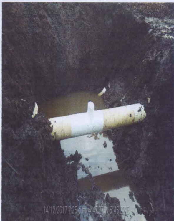
LEAK POINT AFTER REPAIR
